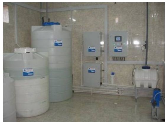
A Chlor-Ozone Plant in Iran
